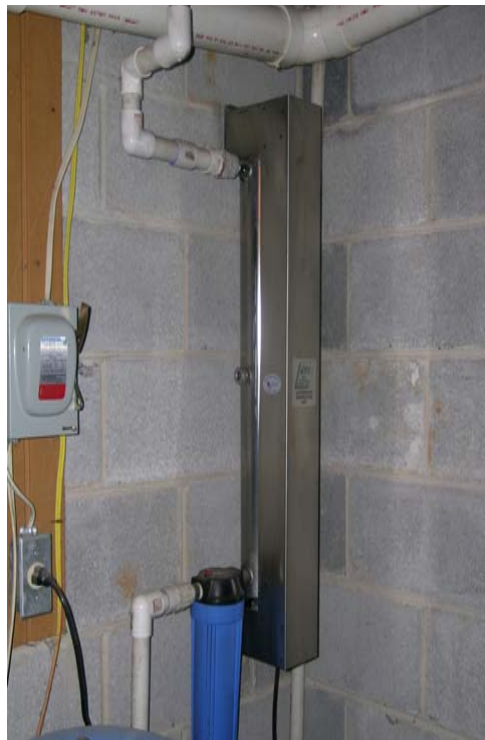
Figure 2. A typical UV light installation with a small canister sediment filter (bottom) ahead of the UV light unit.
